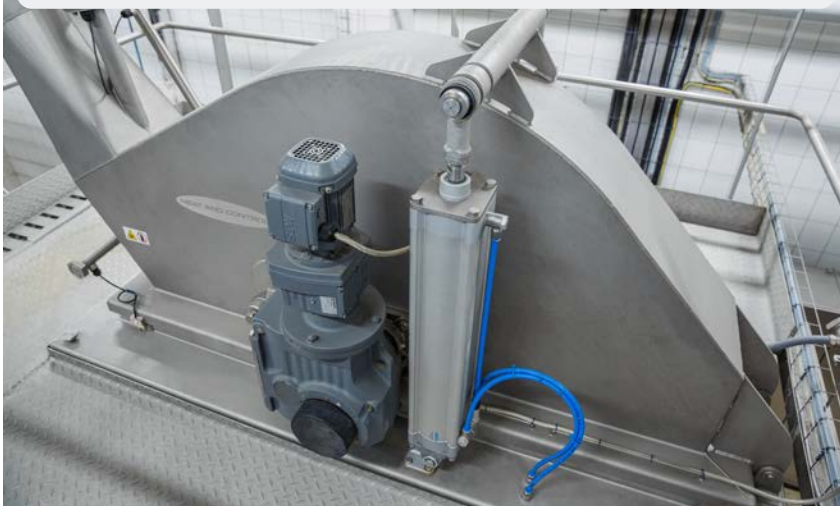
Photo: Heat and Control
